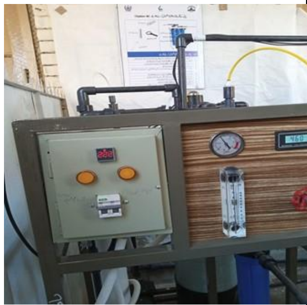
Figure 6: Installed RO system in Govt. Shuhda-E-APS Memorial High School, Sahiwal
